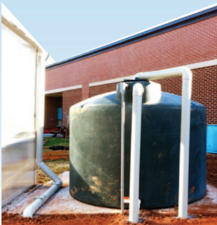
1,500 Gallon Above-Ground Tank
