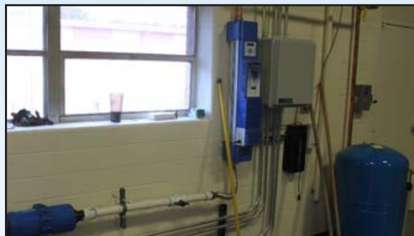
Indoor filtration system
