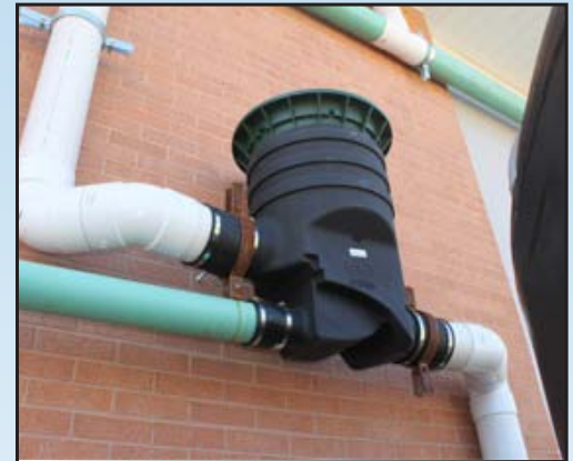
Above ground pump system
