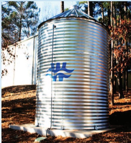
9,200 gallon rainwater collection tank
