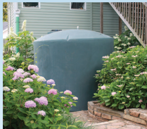
Above Ground Collection System
