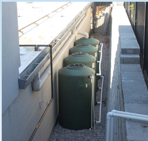
Above ground active collection system
